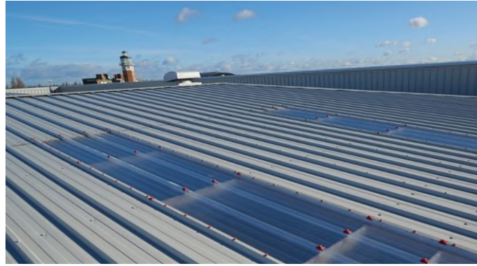
Figure 5. Example of installed roofing panels featuring trapezoidal crowns (visible as ribbing running down the length of the panel).
